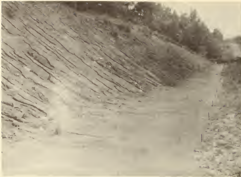
Figure 7.--Soil deposits were 8 inches deep in the upper end of the flow channel, as shown in the foreground of this photograph. The rilled effect of the bank surface was caused by runoff during one rain that followed severe frost action. Later, all the loose soil was washed from the bank, leaving it relatively smooth and firm.
